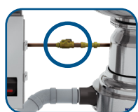
Cold Water Solenoid Valve plumbed to Disposer
